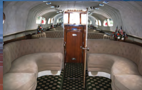
Thunderbird 's bottom is refurbished and interior replaced at Svendsen's Boat Works in Alameda, California.
